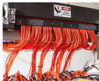
Peristaltic Pumping System
